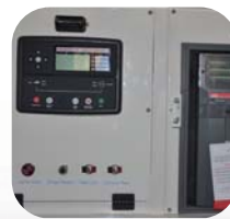
Control Panel & MCB
